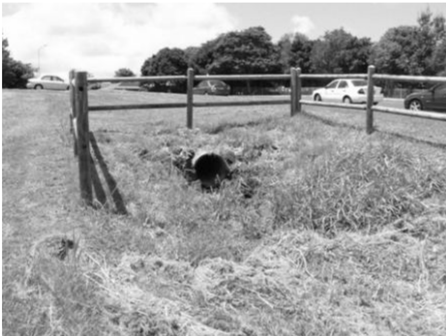
Plate 12: Stormwater pipe in elevated position near Southern Cross School - suitable for a constructed wetland treatment system
