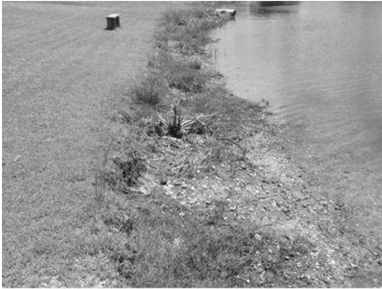
Plate 6: Erosion area along the foreshore bank at Chickiba Lake.
