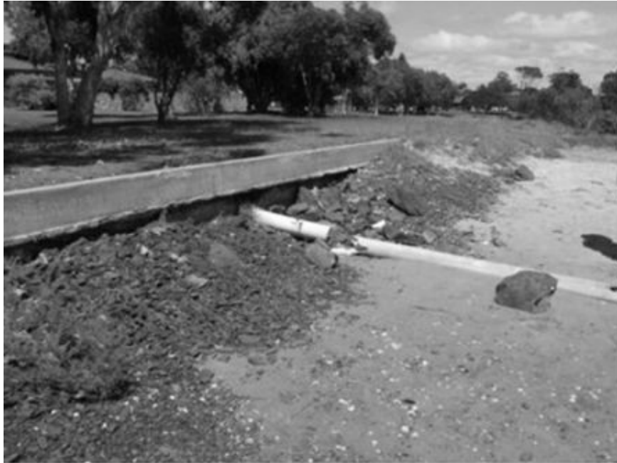
Plate 10: Stormwater pipes discharging into Prospect Lake
