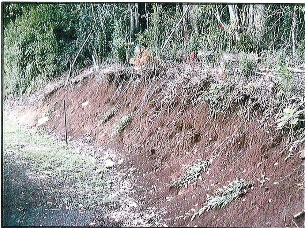
Photo 1: Erosion and Privets
