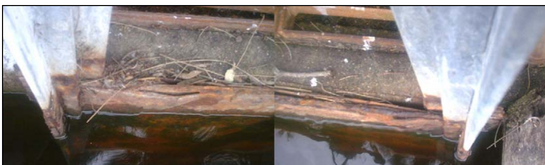
Looking down at the emergency discharge sluice gate which has become rusted closed over the past few years.
