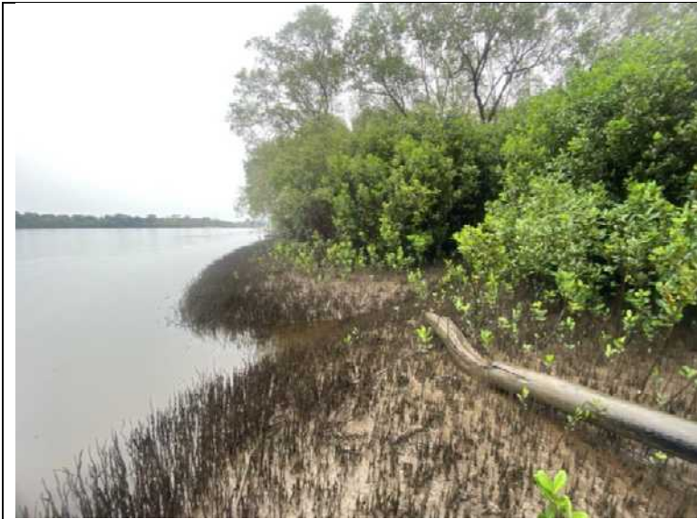
Plate 4. Drain outlet at Richmond River with low growth of River Mangrove and emergent Grey Mangrove
