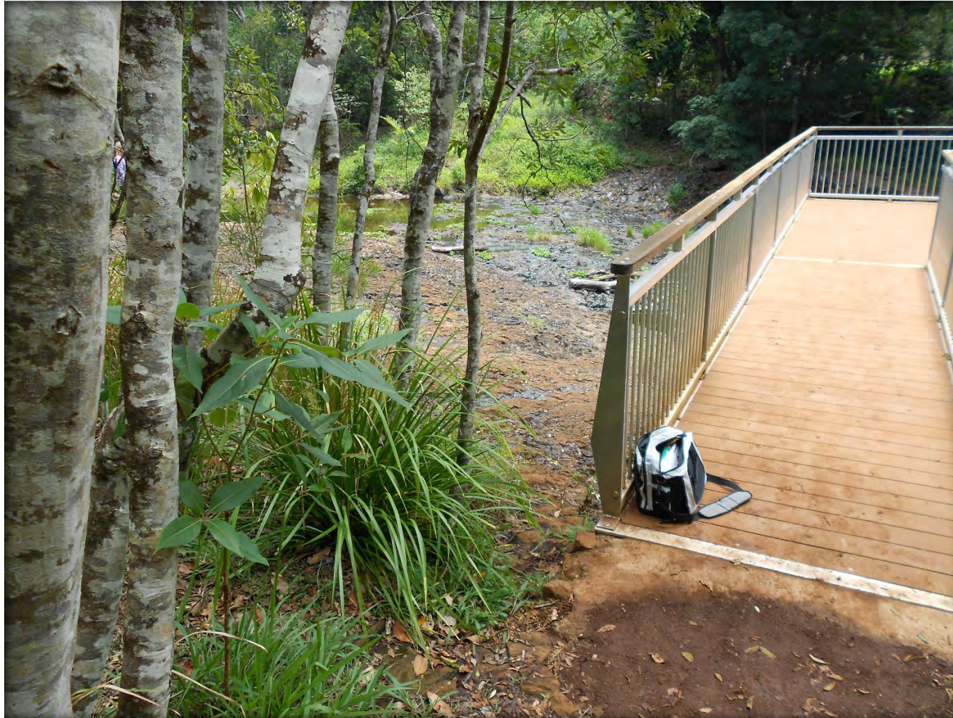
Figure 3: This gap next to the viewing platform needs to be fenced and signposted
