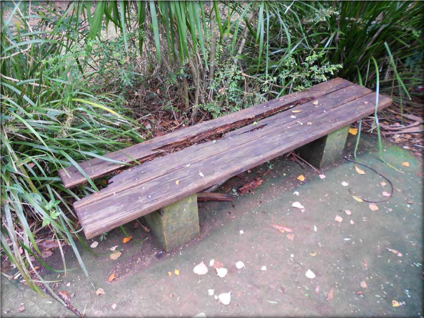
Figure 7: Replace rotten top on existing seat
