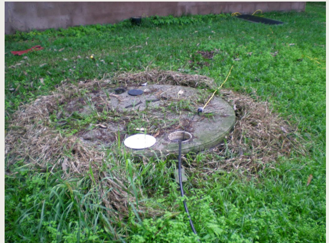
Image: Poorly maintained septic tank
