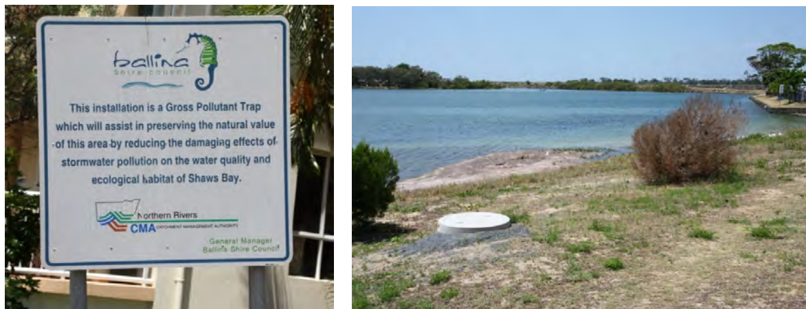
Figure 27: Stormwater GPT installed on western foreshore
