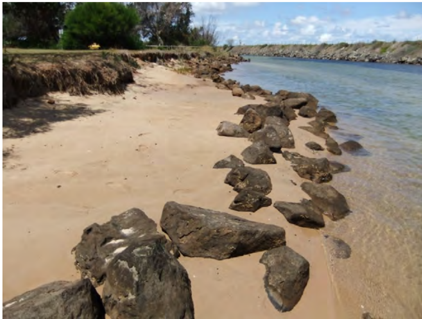
Figure 15: Bank erosion beyond the rock revetment in the East Arm
